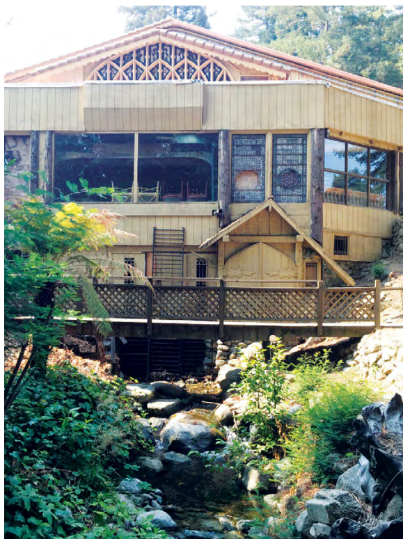
CZU Complex VAR 72. Structure with a channel flowing under it with high debris flow and flooding hazards.
