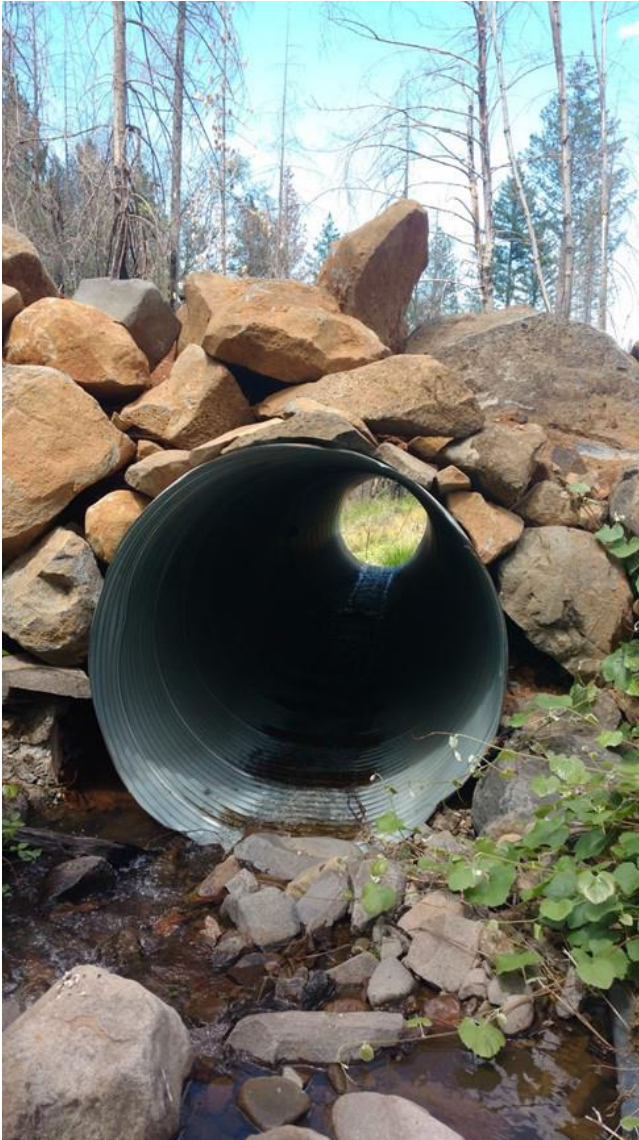
Figure 12. New Class II watercourse crossing at Mill Creek. Two 30 inch culverts were replaced with one 60-inch pipe.
