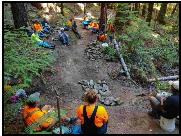
Figure 11. 2023. Rock Ford Trail Crossing – Manly Gulch Trail. Mendocino Coast Cyclists Steam Donkey Crew installing a rocked ford stream crossing.
