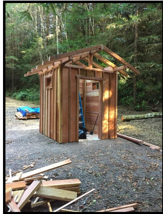
Figure 4. 2019. Outhouse maintenance, Camp 1. JDSF's approach to recreation is rustic, using local materials.
