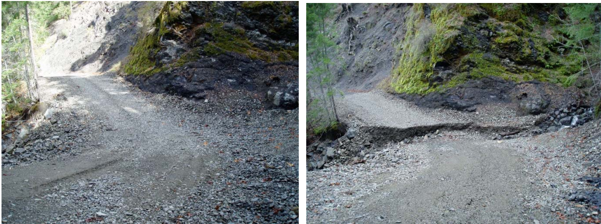
Figure 21. Rock-armed crossing where the outlet rock was undersized, poorly placed, and with insufficient quantity, resulting in post-construction failure. This situation illustrates the need for appropriate sizing of the rock on the outboard edge and close oversight during construction.
