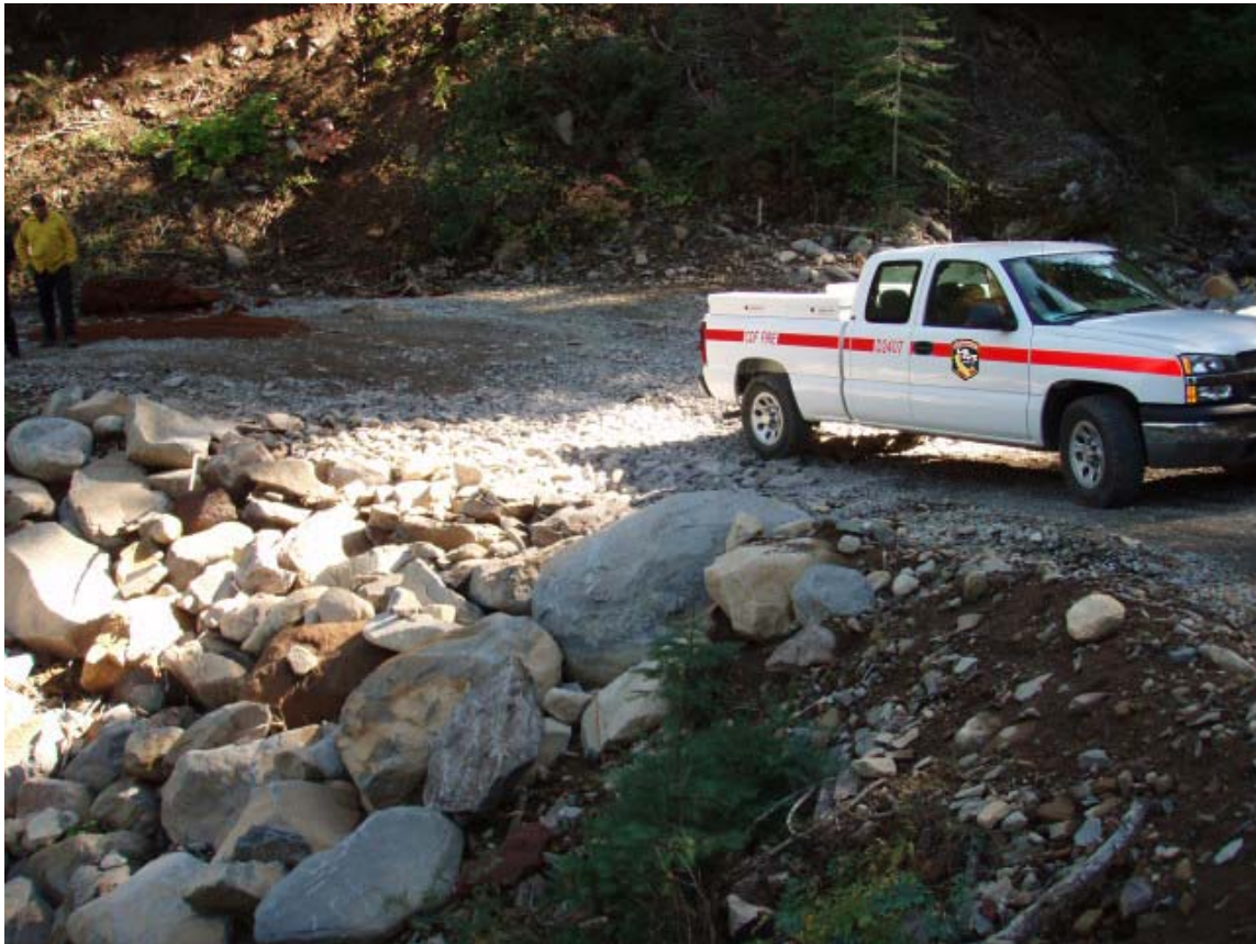
Figure 20. Example of a rock-armored crossing installed in LaTour Demonstration State Forest, Shasta County.
