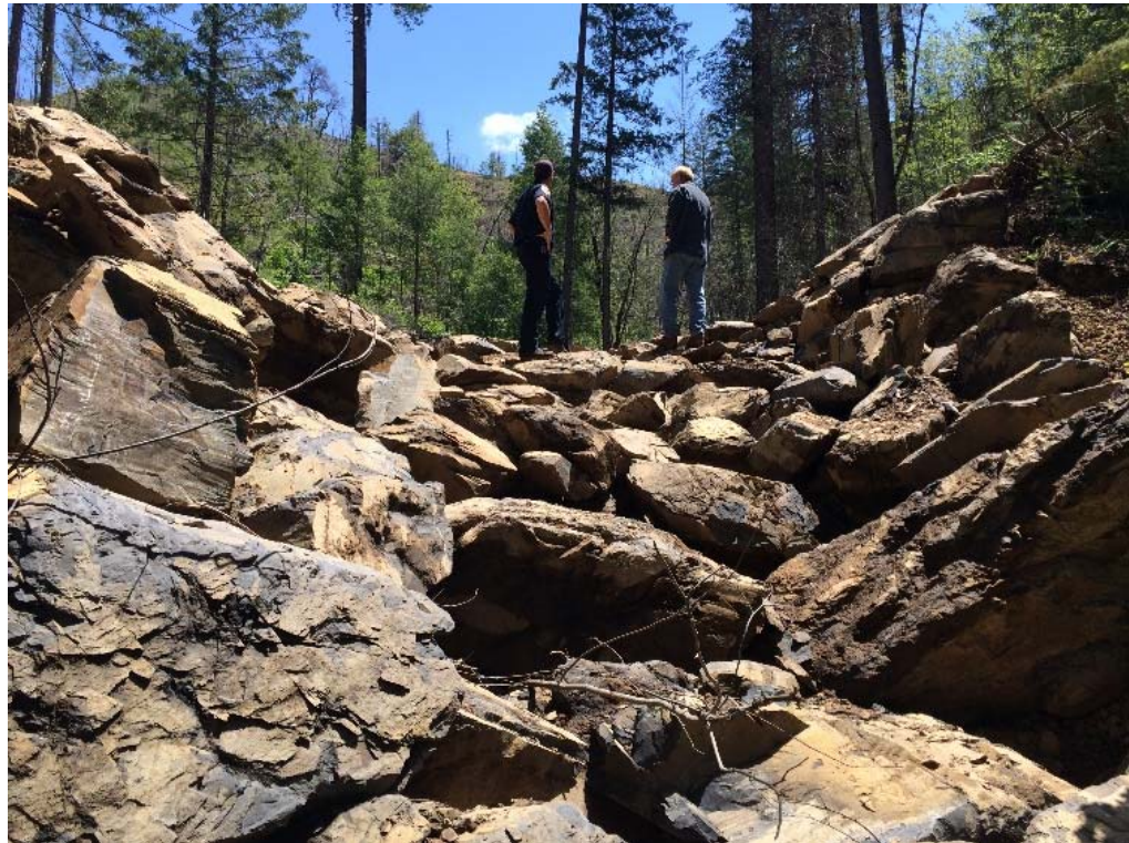
Figure 27. A rock-armed crossing with well-defined armored outfall looking downslope (upper photo) and upslope (lower photo), located in northeastern California.
