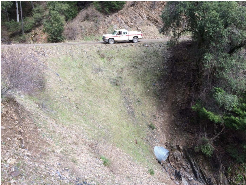
Figure 19. Example of a watercourse crossing with a large fill and a relatively small culvert.
