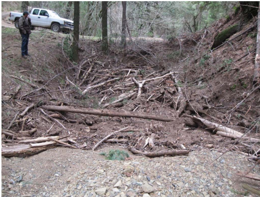
Figure 8. Example of woody debris blocking a culvert inlet following a January 2012 storm event in northern California. The culvert, which is not visible under the debris, is narrower than the channel is wide immediately upstream of the crossing.
