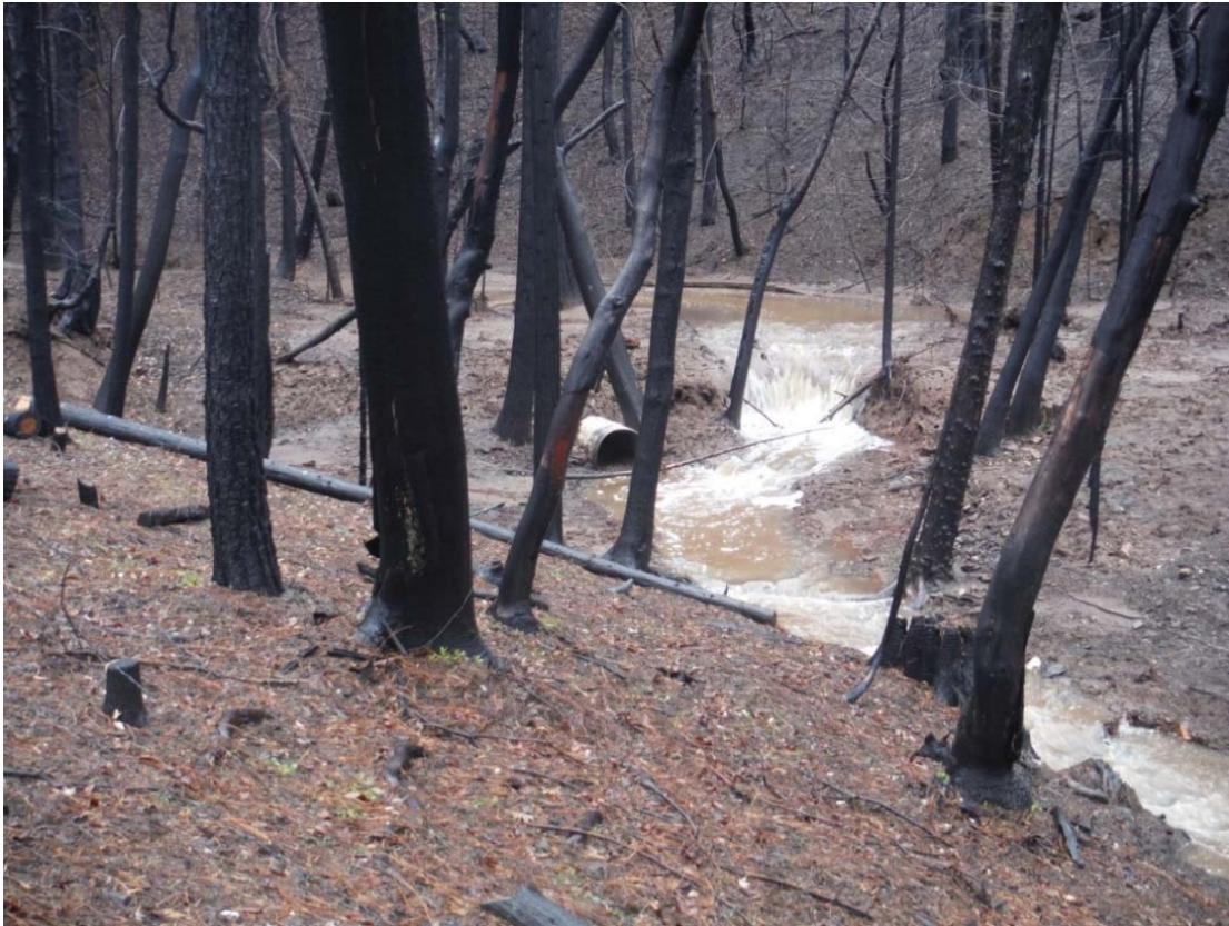
Figure 17. Plugged culvert located in the 2015 Butte Fire area (Calaveras County) during winter storms in March 2016 (photo provided by Cheryl Hayhurst, CGS).
