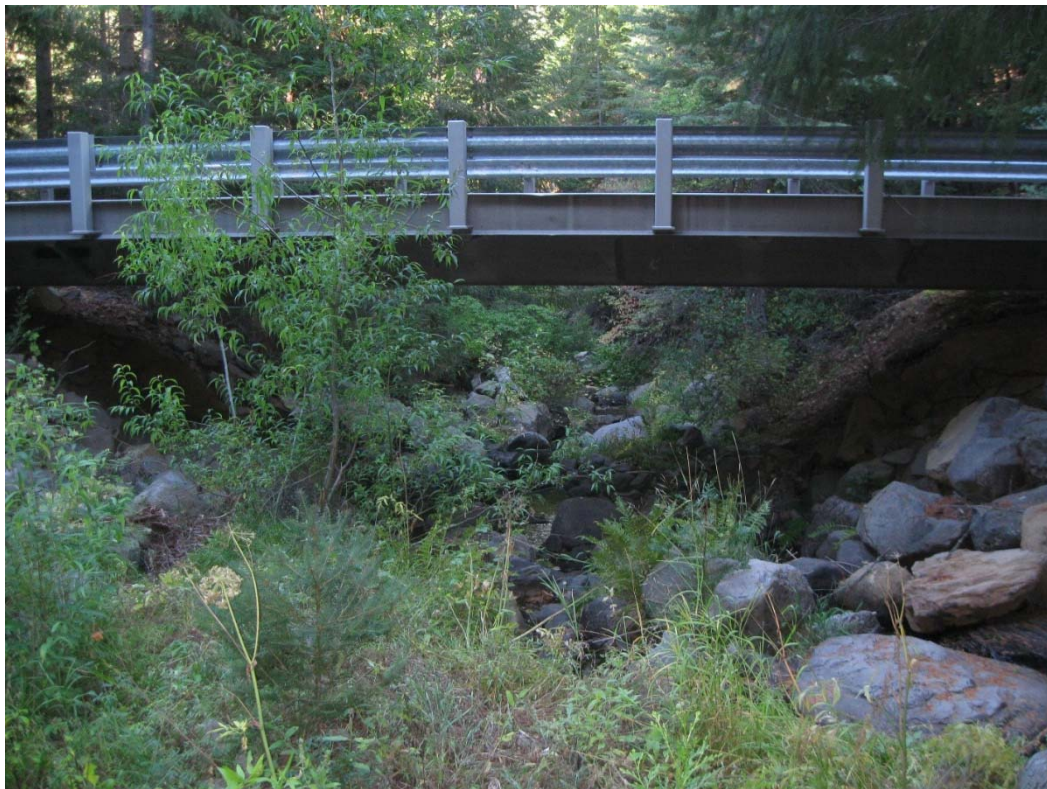
Figure 28. Permanent bridge installed in Shasta County. The bridge spans the entire channel and is positioned above the anticipated flood flow elevation.
