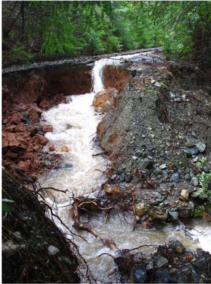
Figure 15. A diverted stream channel caused by a blocked 48 inch culvert in the Six Rivers National Forest (photo from Carolyn Cook, Six Rivers National Forest).
