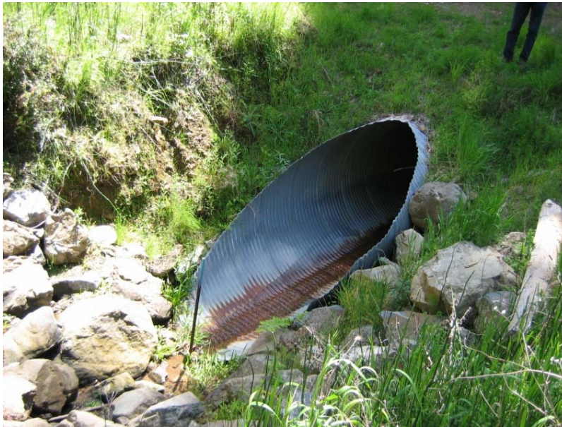
Figure 12. Example of a mitered culvert inlet. This culvert is located in the northern part of the California Coast Ranges.
