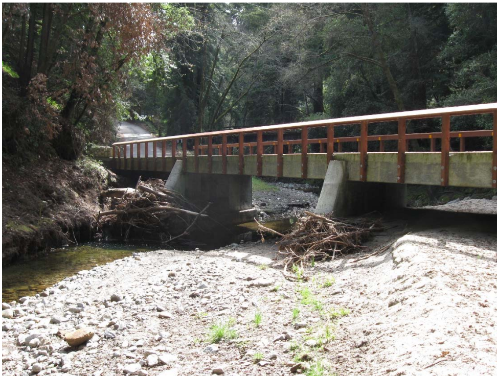
Figure 33. Heavily reinforced concrete bridge with sacrificial wood railings that is designed to be overtopped in the event of a flood event, located in Santa Cruz County.
