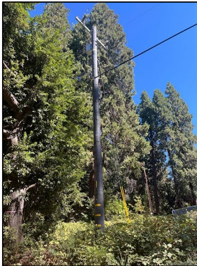
Example of aboveground utility with hazardous vegetation observed during field-based assessments.
