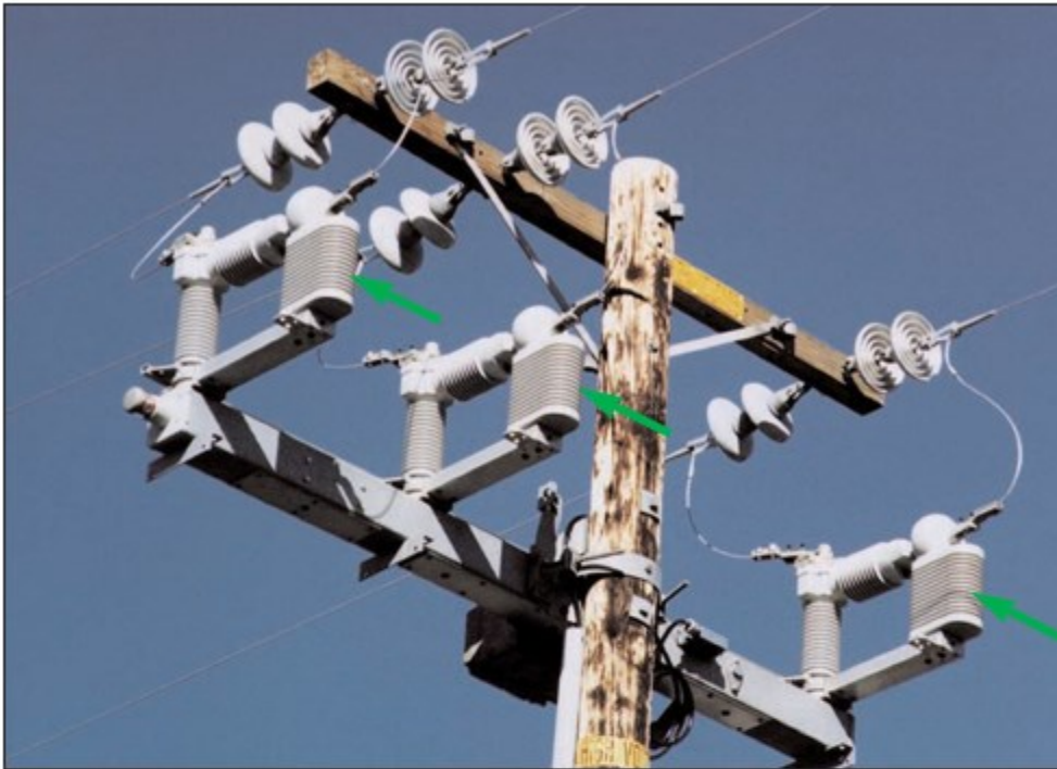
Figure B-37: S&C Scada-Mate Switch
