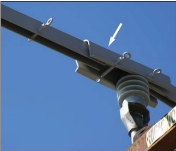
Figure PLC-25: Close-up of Insulator and Wire Cover
