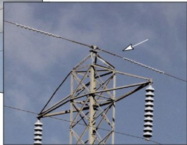
Figure PLC-37: Close-up of Static Line
