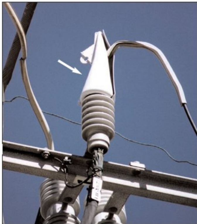
Figure PLC-23: Close up of Squirrel Guard
