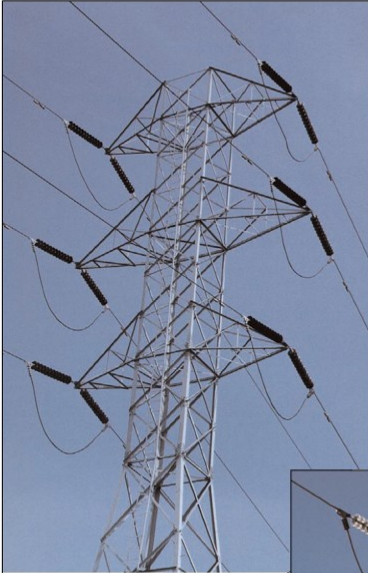
Figure PLC-34: Dead-end Tower
