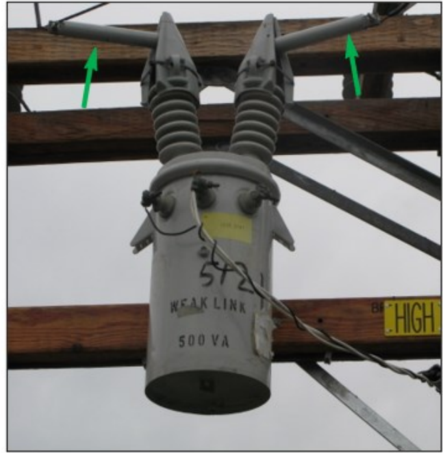
Figure B-5: Hi-Tech Ext/Eaton Cooper Companion II Bushing Mounted Current-Limiting Fuse
