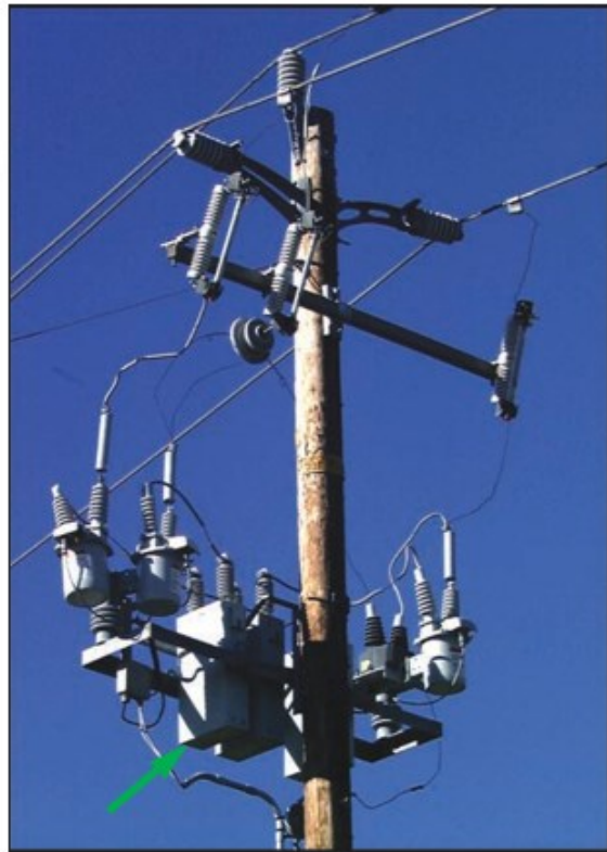
Figure B-51: Capacitor Unit
