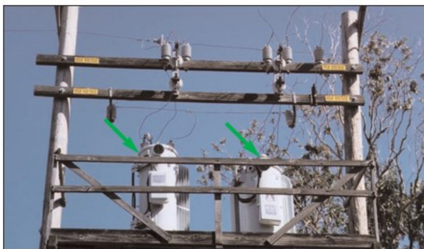
Figure B-49: Voltage Regulator
