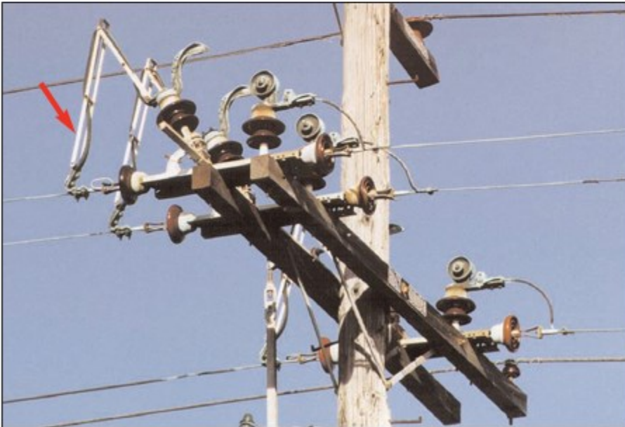
Figure NE-39: Grasshopper Air Switch (open position)
