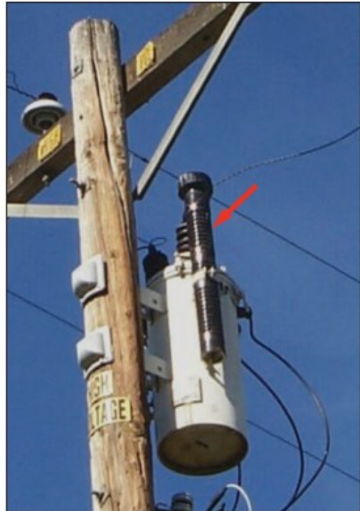
Figure NE-28: Lightning Arrester
