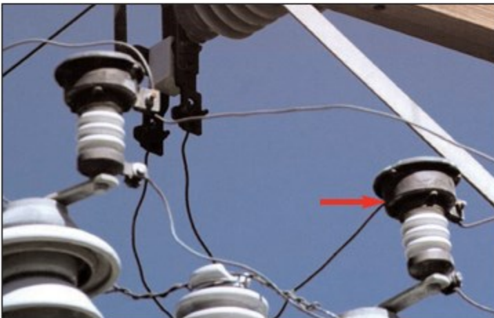
Figure NE-22: Lightning Arrester
