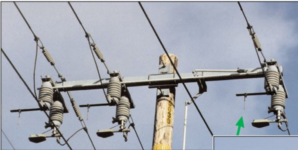
Figure B-26: Eaton-Cooper 600 Amp Underarm Side Break Switch (Open Positions)
