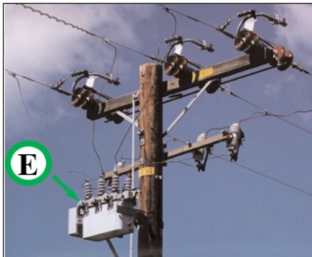
Figure B-45: Sectionalizer with Solid Blade Disconnects
