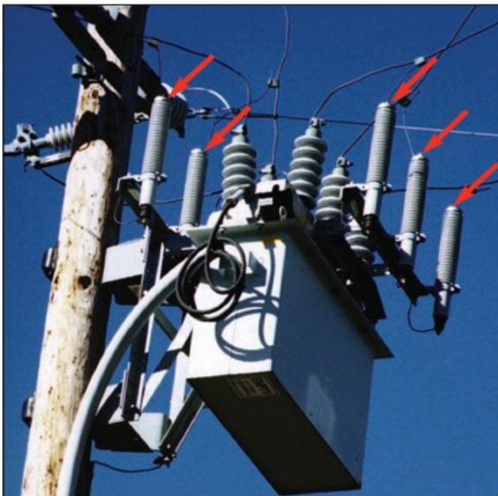
Figure NE-20: Lightning Arrester (with Recloser)
