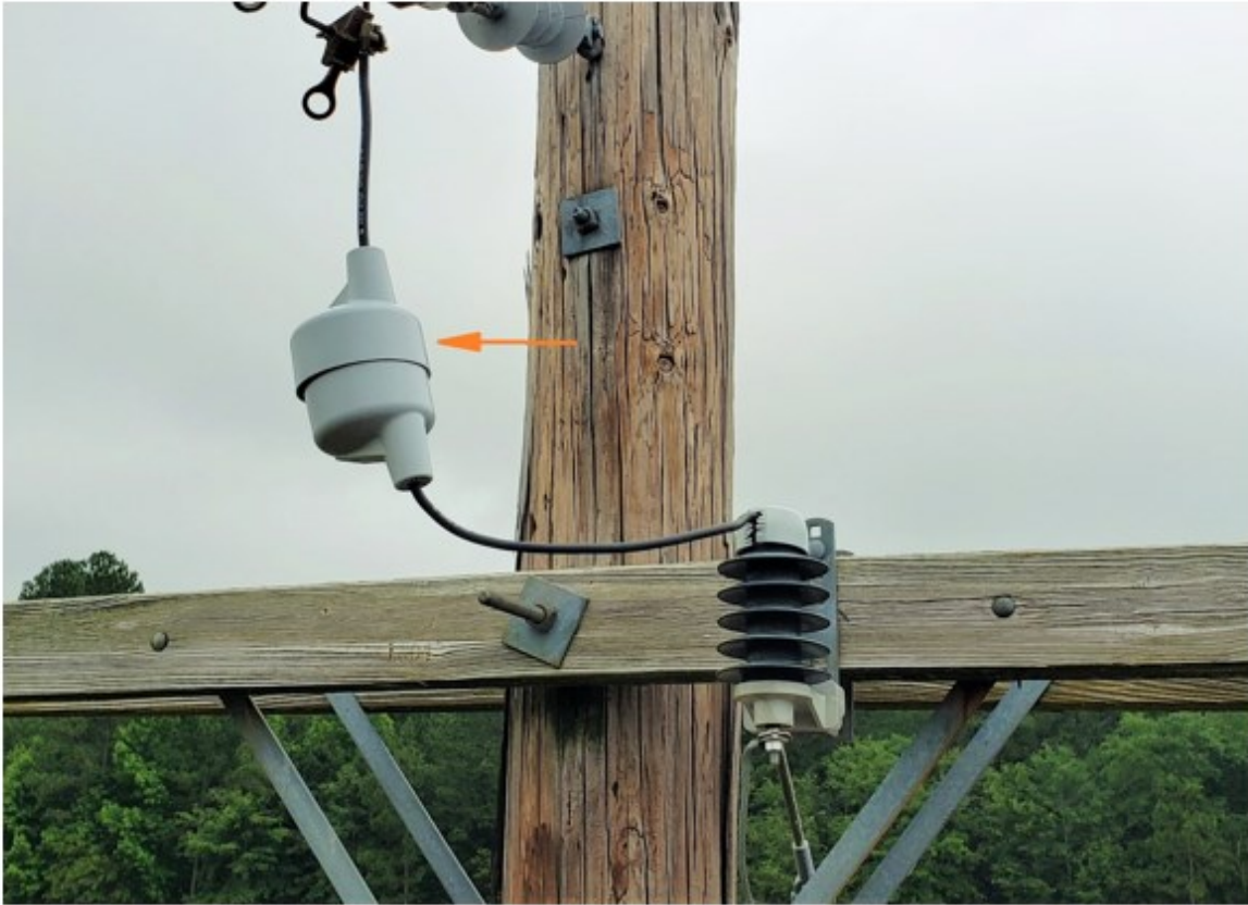
Figure A-1 Hubbell Fire Protection Disconnect Attached to Hubbell Surge Arrestor
