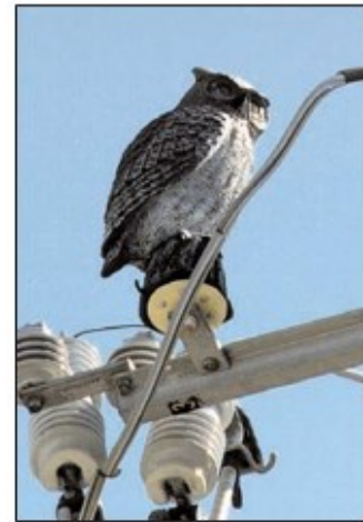
Figure PLC-21: Close-up of Owl on Crossarm
