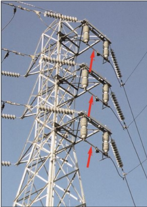
Figure NE-41: Transmission Air Switches Tower Mounted (closed position)
