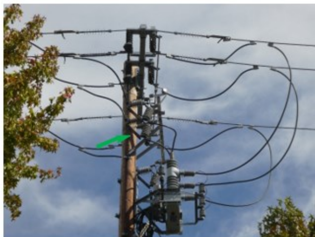
Figure B-47: 600A Disconnect. It is non-exempt equipment as part of recloser installation
