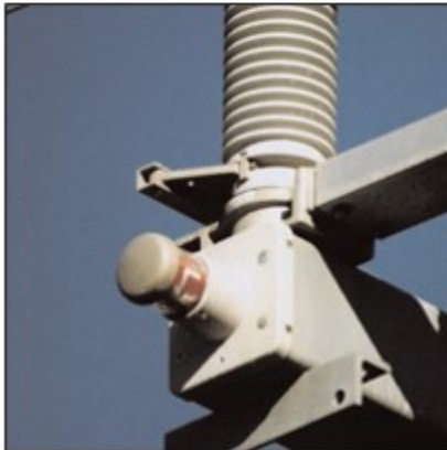
Figure B-39: Closed Position Indicator Red
