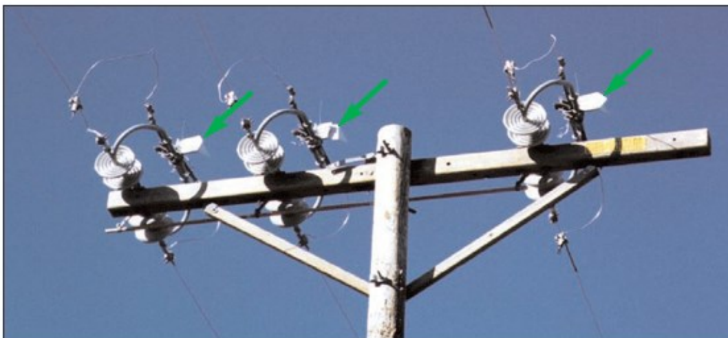
Figure B-24: 600 Amp KPF Air Switch, Crossarm Construction (Closed Position) with Arcing Horns and Snuffers
