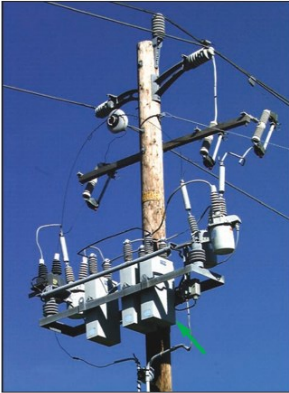
Figure B-50: Capacitor Bank
