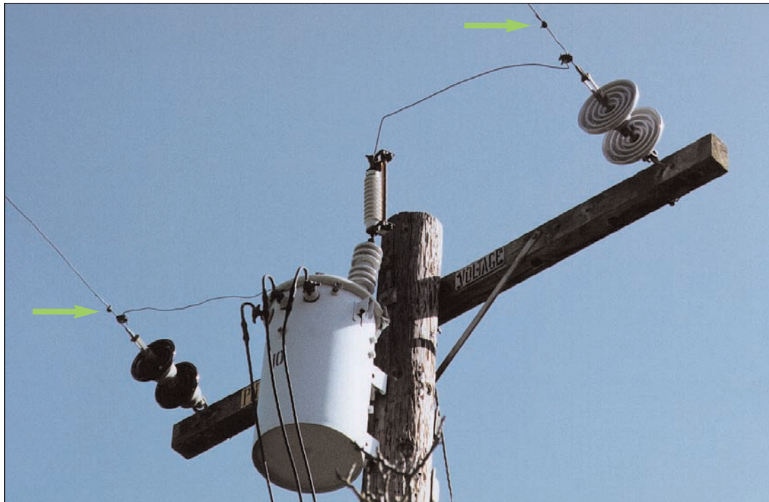
Figure 3-57 Idle Split Bolt Connectors
