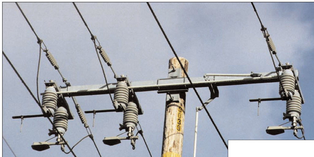
Figure 3-24 600 Amp Underarm Sidebreak Switch (open position)
