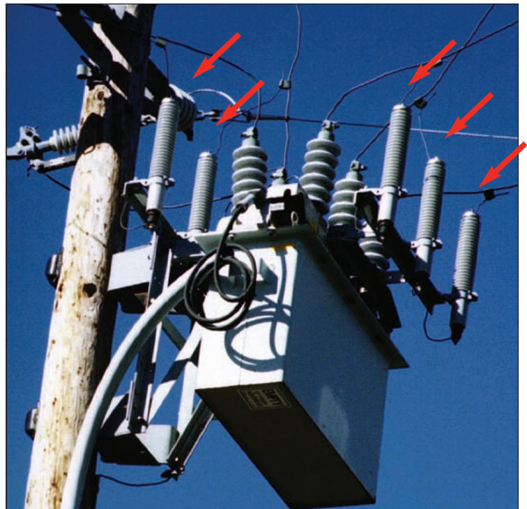
Figure 2-20 Lightning Arrester (with Recloser)
