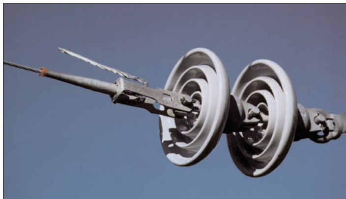
Figure 3-68 Automatic Deadends with Suspension Insulators
