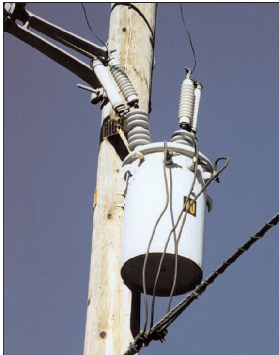
Figure 3-5 Bushing Mounted Cutout with Non-Expulsion Fuses
