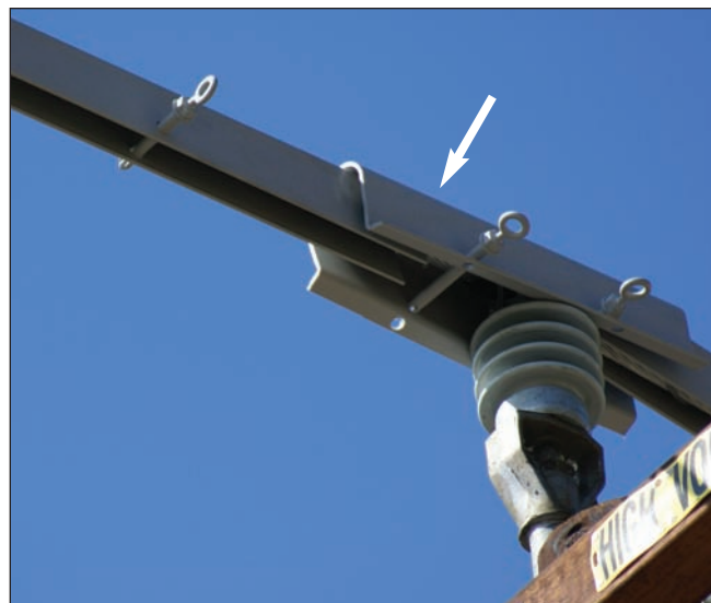
Figure 4-23 Close up of Insulator and Wire Cover
