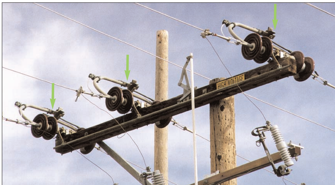
Figure 3-23 600 Amp KPF Air Switch, Crossarm Construction (closed position) without Arcing Horns or Snuffers
