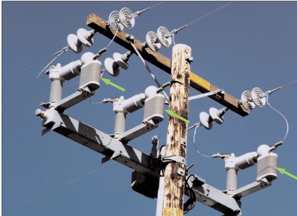
Figure 3-33 S&C Scada-Mate Switch
