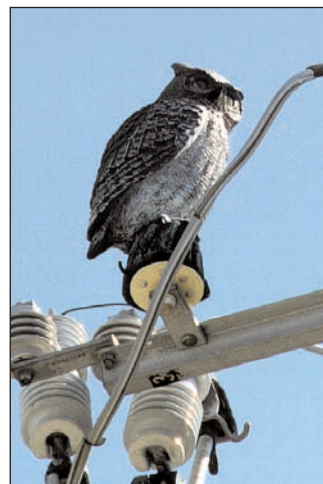
Figure 4-19 Close up of Owl on Crossarm
