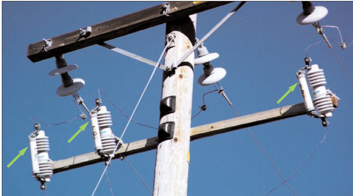
Figure 3-3 Arm Mounted Cutout with Non-Expulsion Fuses
