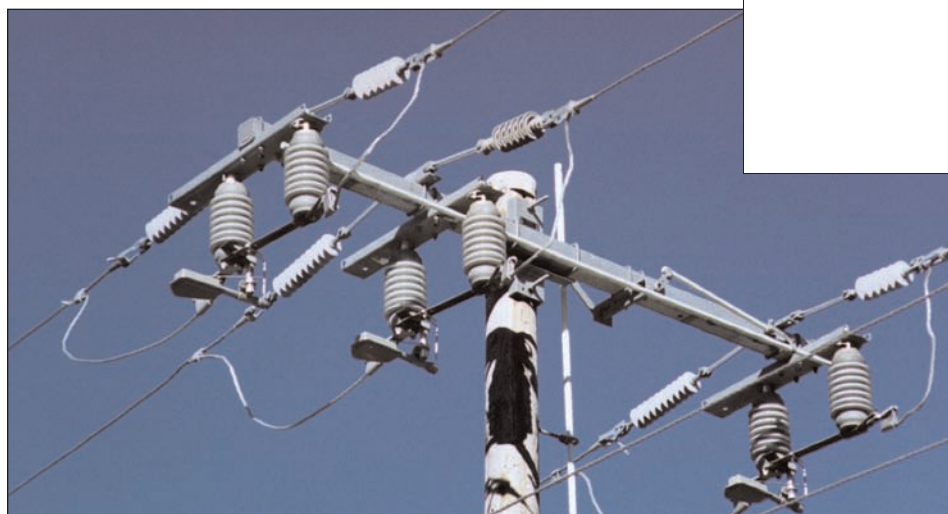
Figure 3-27 600 Amp Underarm Sidebreak Switch (closed position)
