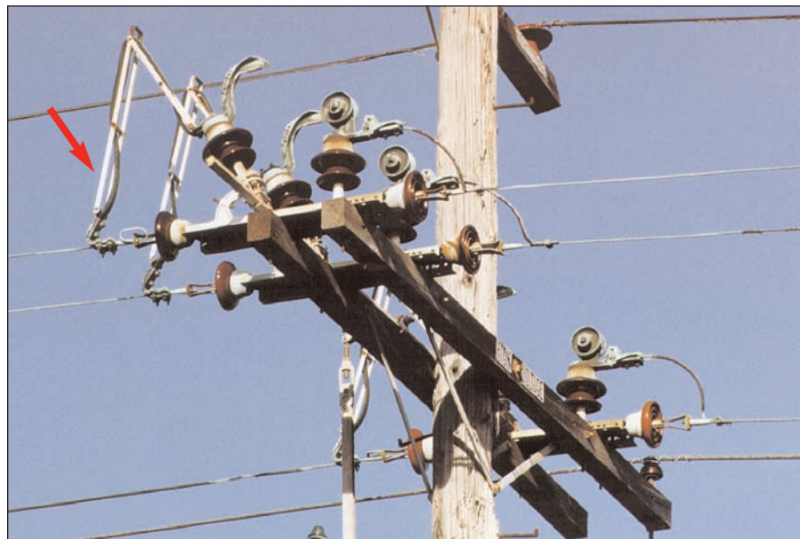
Figure 2-39 Grasshopper Air Switch (open position)
