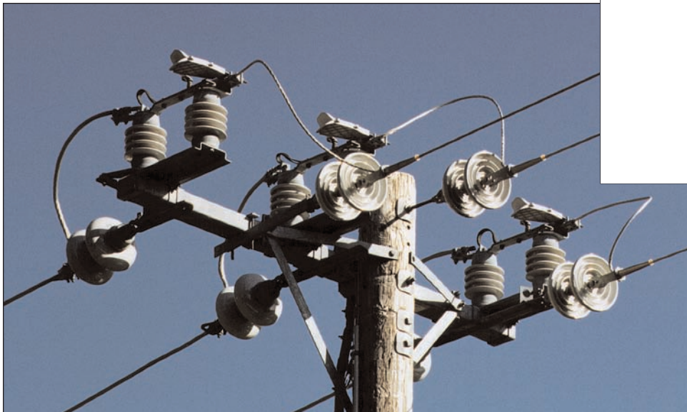
Figure 3-31 S&C Omni-Ruptor Switch, Tangent Construction (closed position)
