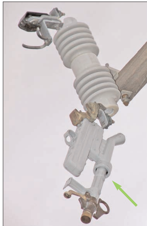
Figure 3-19 S&C Fault Tamer Fuse (Open)
