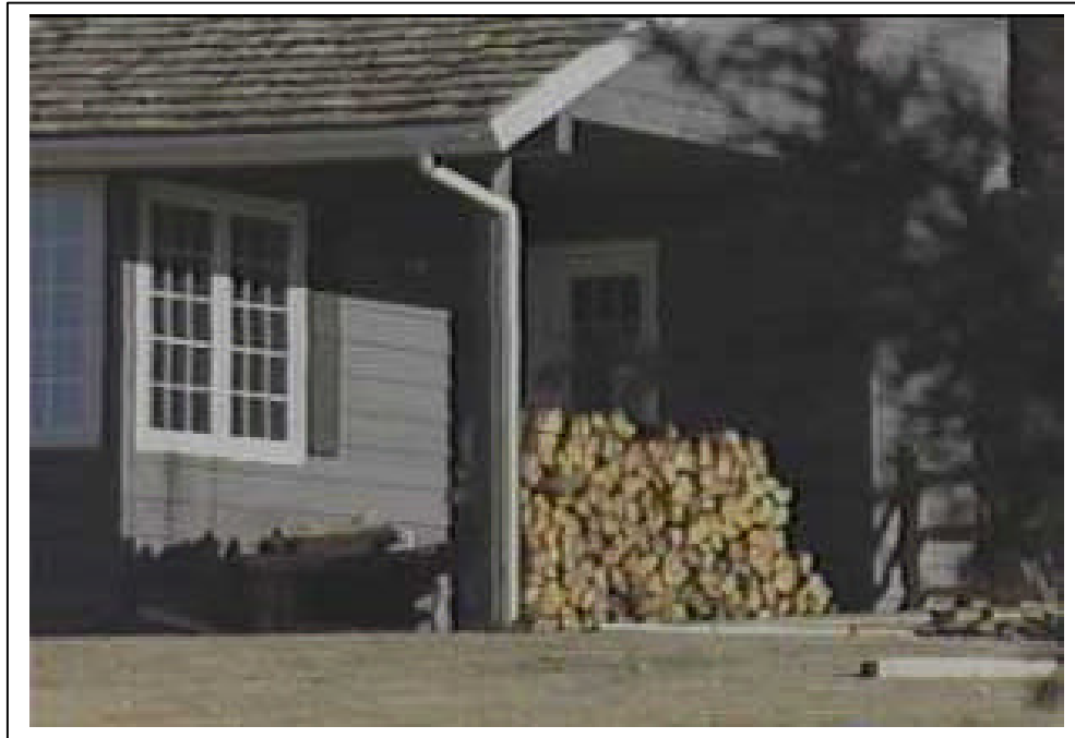
Photograph 12.3. Improper Placement of Firewood
